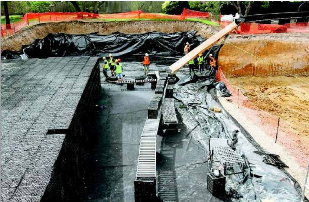
Above: recycled plastic crates will be used in a 4.6 million litre water storage under Jacka Reserve in North Balwyn.
