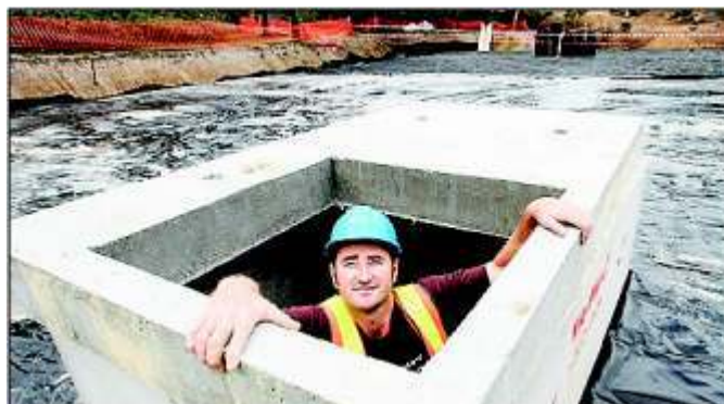
Right: the director of tank installer Sub Terra, Peter O'Neill, in the inspection well in North Balwyn.
